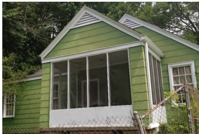
Housing unit repaired through the Lead Safe Jackson Housing Program, where lead paint hazards were identified in the screen porch and child's outdoor play area.
