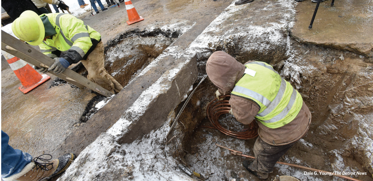
Lansing Board of Water and Light employees replace the last lead service line with copper pipes in Lansing, Michigan, on Dec. 14, 2016.
